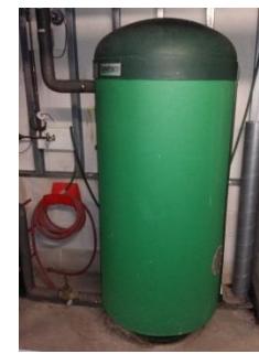
boilervat warm tapwater
